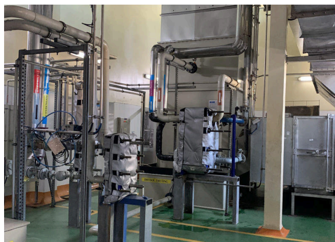
Equipment from our Dutch partner installed and operating at a plant in Vietnam. Kim Nguyen archive photo.
