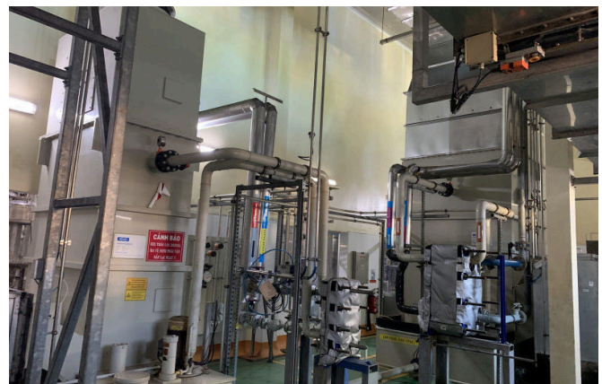
Gelatine plant – drying equipment and steam piping, made in the Netherlands, after installation. Kim Nguyen archive photo.
